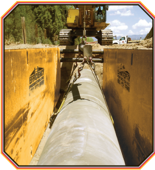
steel trench shield
